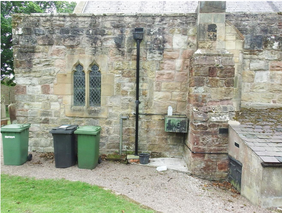
The east end of the chancel aisle from the north; note blocked window (behind drainpipe) which is cut across internally by the wall that divides the former vestry from the remainder of the aisle
