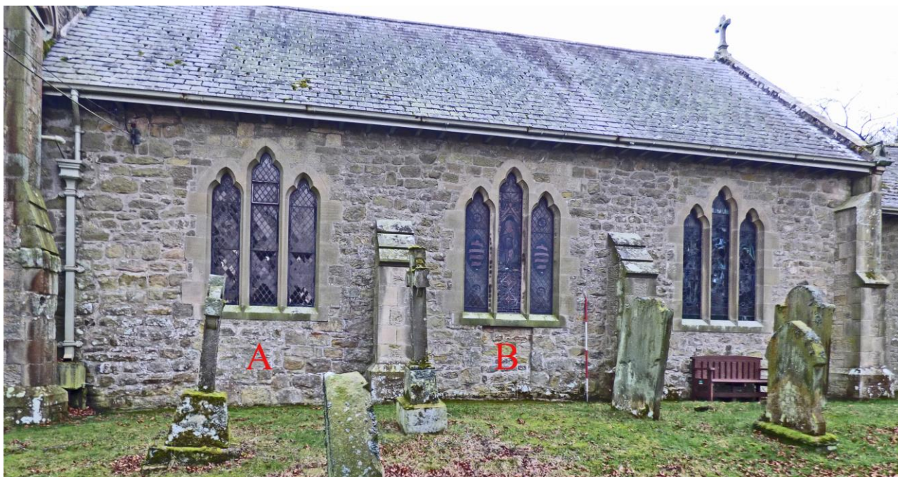
South nave wall: the two blocked doorways are labelled A and B
