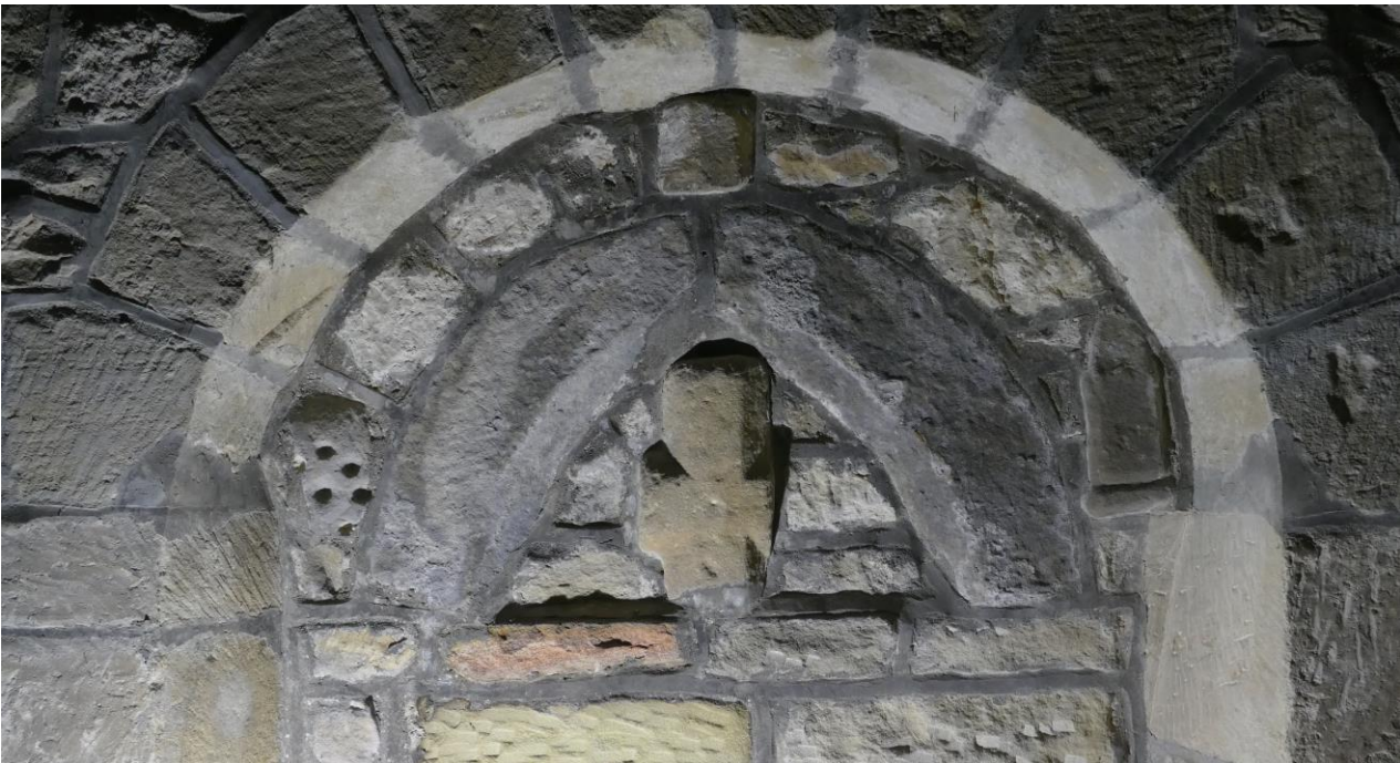
The recess of the blocked priest's door, with various architectural fragments re-set in 1884
