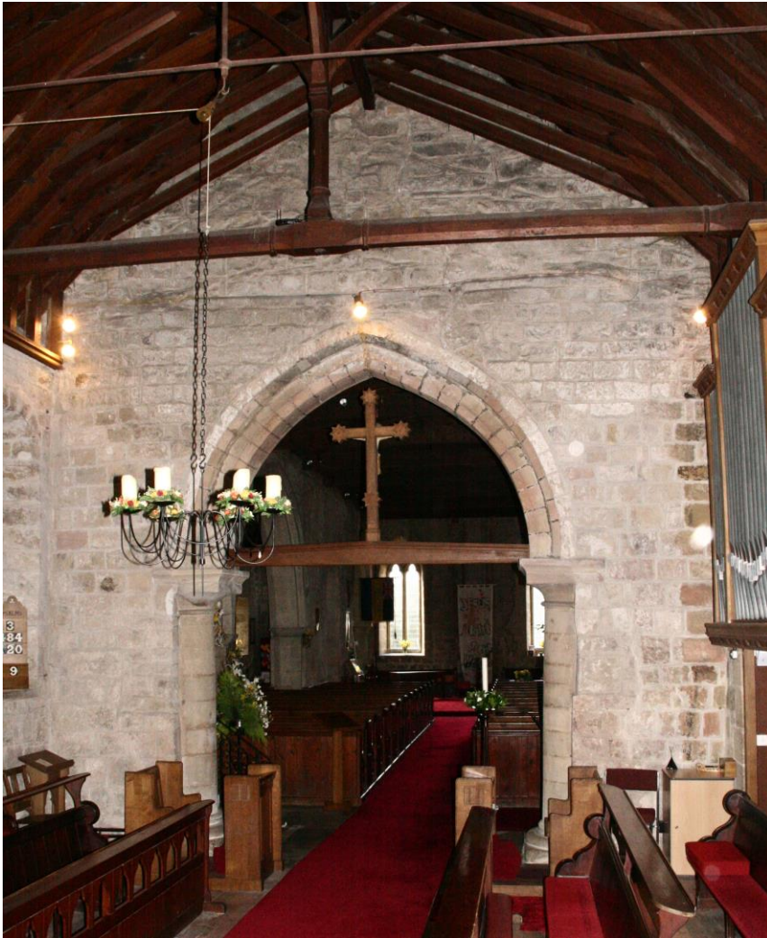
The chancel looking west; Note patched masonry in jambs of arch, and evidence of two earlier roof-lines
